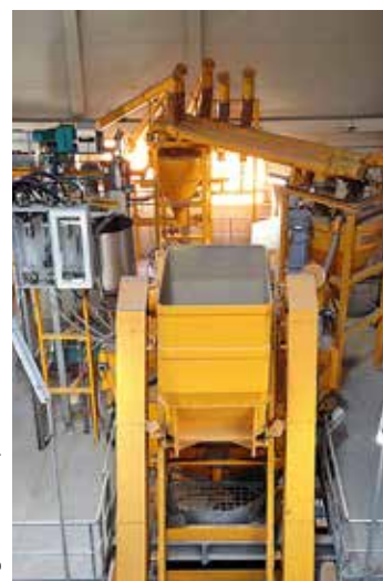
Detail view of the MCT Mixer floor
