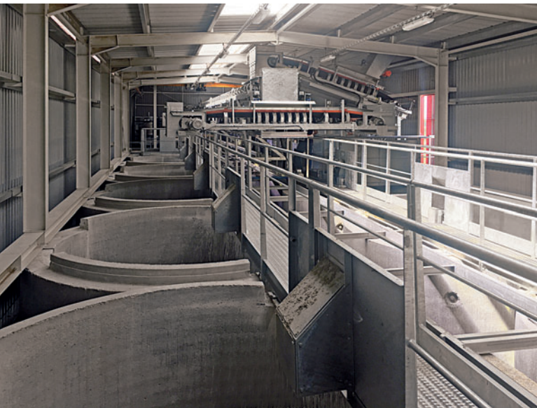
Aggregate dispensing platform on the top of the storage
