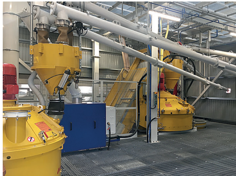
View of the mixers platform
